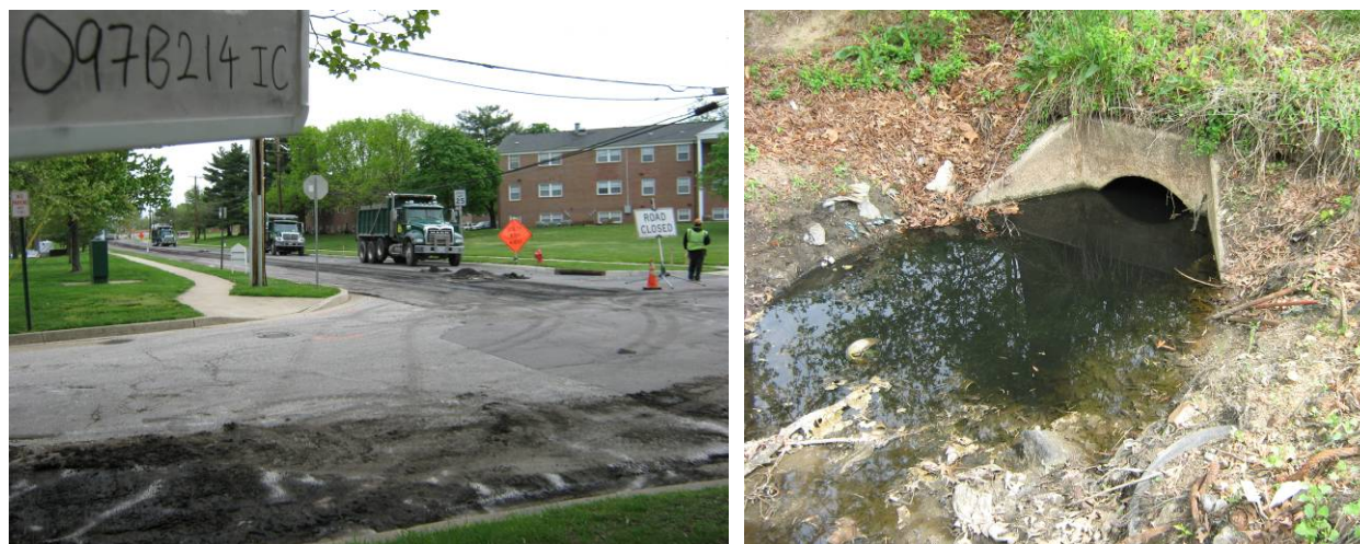
Figure 3-24: Severe Near Stream Construction at the End of Mansfield Road
