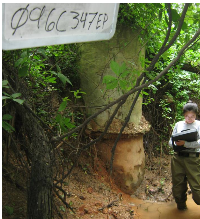
Figure 3-21: Examples of a Potentially Severe Exposed Pipe Problem (rating = 2)
